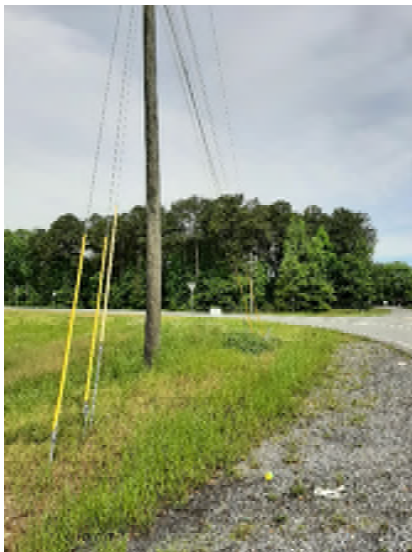
Electrical lines (SW quadrant of intersection)
