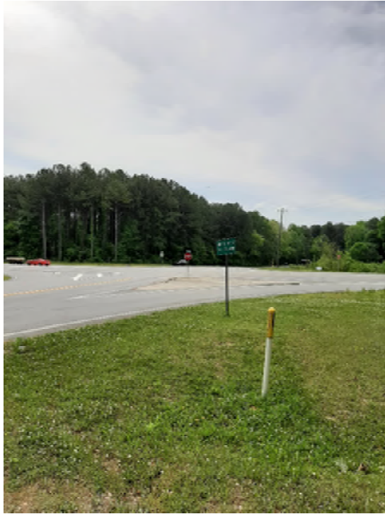
Gas line (NW quadrant of Intersection)
